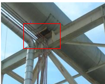
Gambar 2. Pergeseran Saddle Support Pipa Transfer Line
