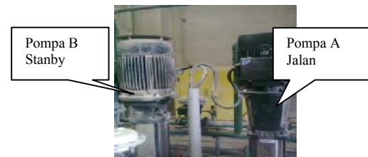
Gambar 4.2 Pompa Air Cooling Tower
