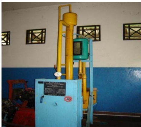
Gambar Hydraulic Engine Test Bed
