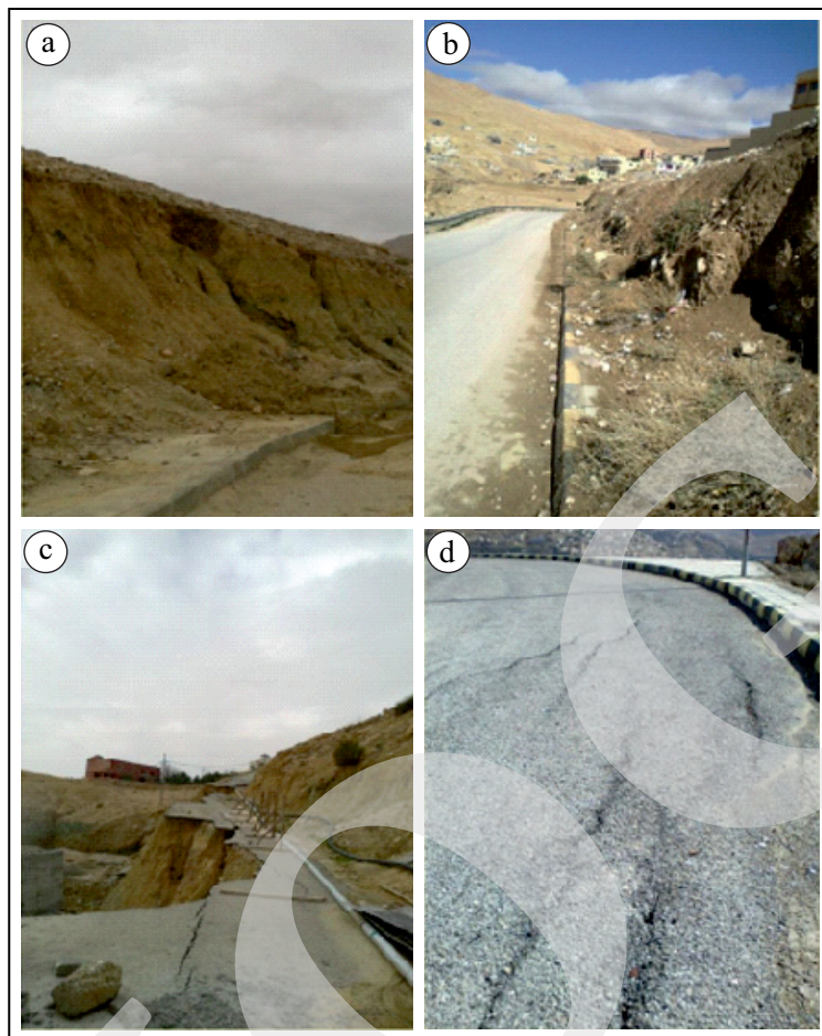
Figure 5. Registered landslides (a, c) and erosions (b, d) in the streets and roads of the studied area.
