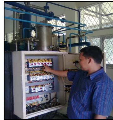
(4.c) Instrumen Panel Boiler
